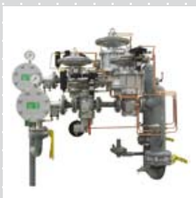
Reducing and metering stations
