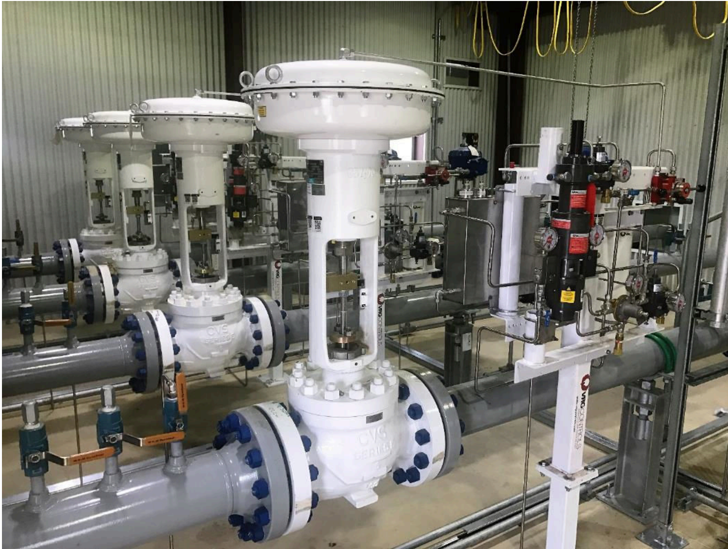
Louisville Gas & Electric (LG&E) CVET Globe Control Valves with VPC Valve Pilot Controllers w/ VMO
